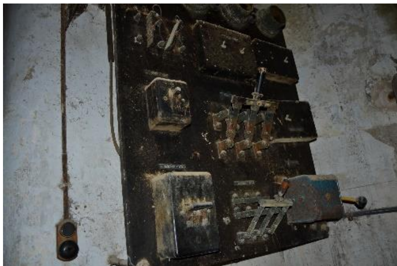
Electrical table of the old machine 150
